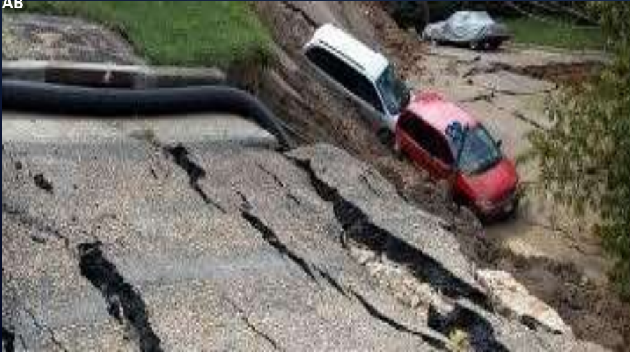
Landslide Impacted Area: See and measure, support to immediate analysis
