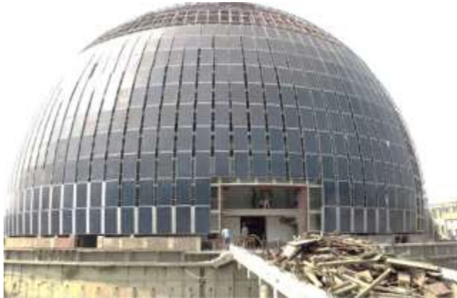
a photovoltaic dome (Diameter 45m, Height 27m)
