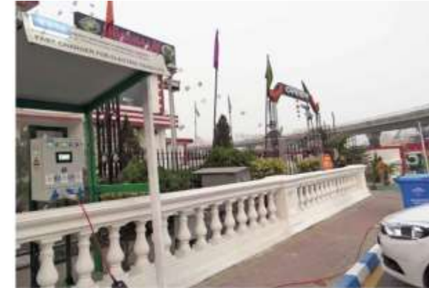
Electric vehicle charging facilities
